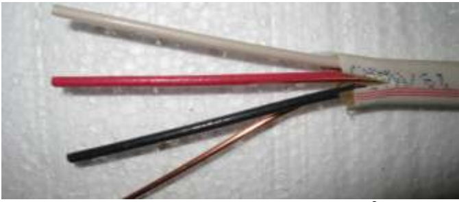
This picture above shows the end of a 14-3 with ground, 2 hots, white neutral and bare ground.
